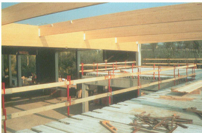
Fig. 4-3: Glue laminated beams and rafters provide the roof to a precast concrete supermarket structure. (Courtesy of Ergon, Belgium)
