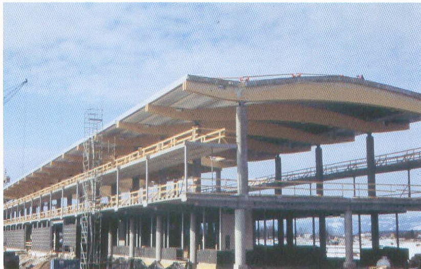
Fig. 4-5: Glue laminated timber rafters supported off precast concrete columns at Oslo International Airport. (Courtesy of Spenncon, Norway)
