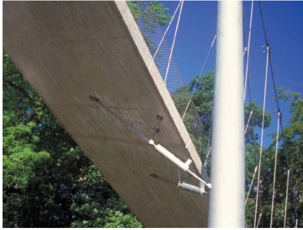
Fig. 5.23 Example of viscous damper on the footbridge in Minden, Germany. Viscous damper installed between pylon and deck slab
