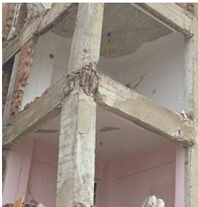
b) Detailed view of beam-column joint damage
