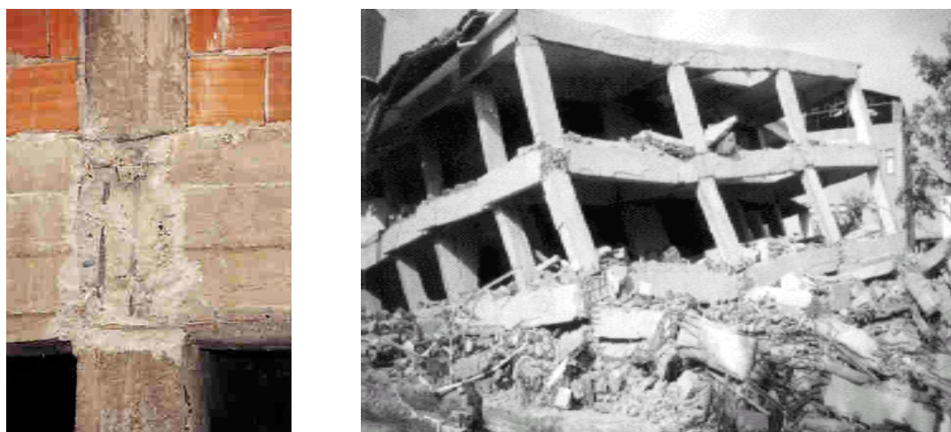
Fig. 7: Failure of beam-column joints
