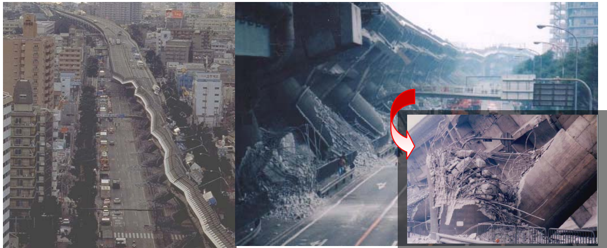
Fig. 10-5: Flexural failure above column base of columns of the Hanshin expressway, due to premature termination of longitudinal reinforcement and inadequate confinement in the 1995 Kobe earthquake (courtesy of Kawashima). (Figure available electronically on fib website; see production note on p. ii)
