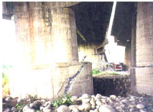
Fig. 8-4: Wushi Bridge - settlement and shear cracks at pier P3N
