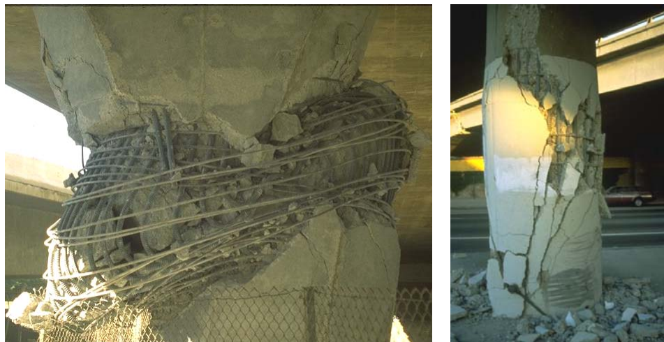
Fig. 10-6: Shear failure within (left) and outside (right) the plastic hinge region in San Fernando Mission Blvd-Gothic Avenue Bridge and I-10 Freeway at Venice Blvd, respectively, during the 1994 Northridge earthquake (after NISEE, 2000). (Figure available electronically on fib website; see production note on p. ii)
