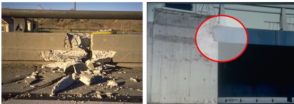
Fig. 10-3: Pounding damage: between adjacent spans at the Interstate-5 at Santa Clara River in Los Angeles County during the 1994 Northridge earthquake (left) and at the abutment of a bridge near Nishinomiya Port in the 1995 Kobe earthquake (after NISEE, 2000). (Figure available electronically on fib website; see production note on p. ii)
