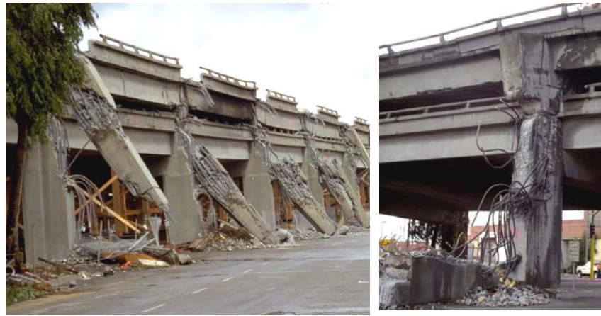
Fig. 10-8: Sliding shear at top columns of the Cypress viaduct in the 1989 Loma Prieta earthquake (after NISEE, 2000). (Figure available electronically on fib website; see production note on p. ii)
