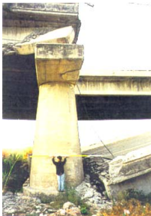
Fig. 8-2: Wushi Bridge - span collapse due to longitudinal movement at pier P2N
