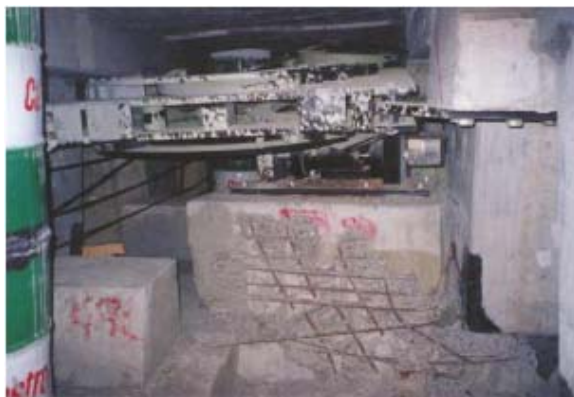
Fig. 8-7: Bolu Viaduct - failure of an EDU
