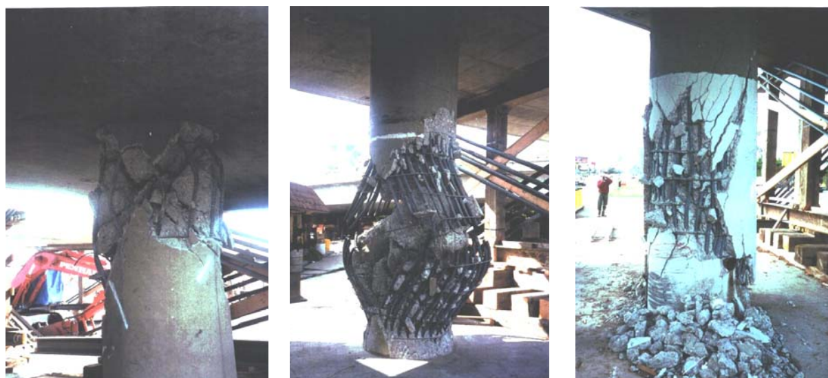
Fig. 10-7: Different shear damage patterns for RC piers at the under-crossing of the Santa-Monica Interstate 10 during the 1994 Northridge earthquake: Piers # 5 with inadequate detailing for plastic hinge (left), Piers # 6 with symmetric buckling (middle) and Pier # 8 with typical shear failure (right) (after Broderick et al. , 1994). (Figure available electronically on fib website; see production note on p. ii)
