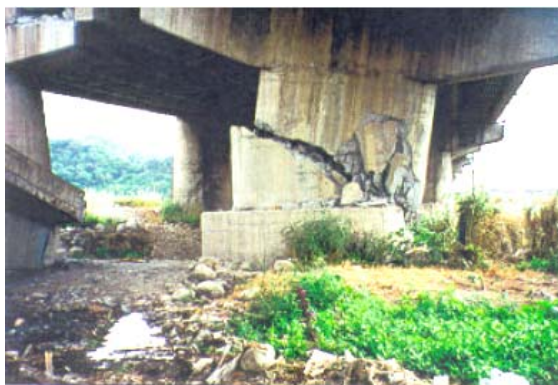
Fig. 8-3: Wushi Bridge - shear failure of pier P2S
