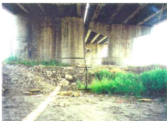
Fig. 8-1: Wushi Bridge - fault movement between piers 2 and 3
