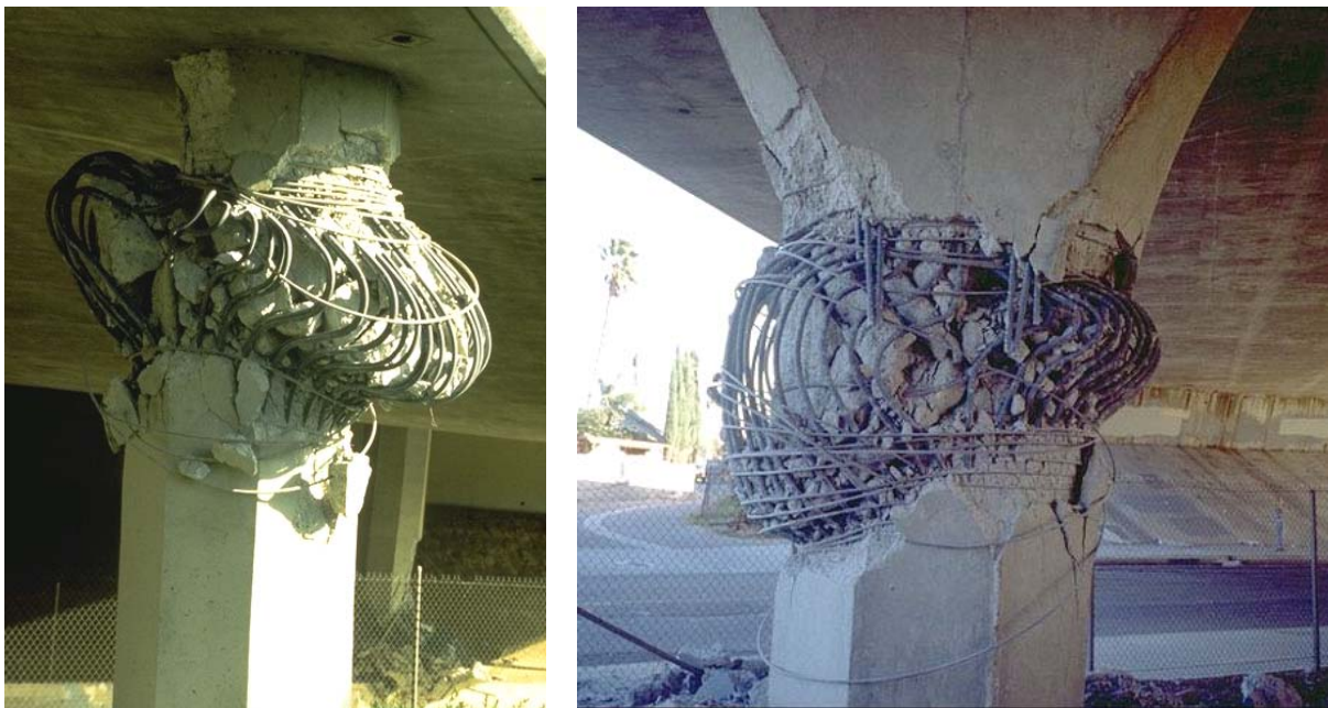
Fig. 10-4: Confinement failure at bridge pier top during the 1994 Northridge earthquake (after NISEE, 2000). (Figure available electronically on fib website; see production note on p. ii)
