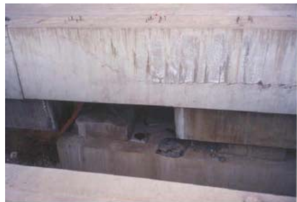
Fig. 8-8: Bolu Viaduct - unseating of beam end at pier cap
