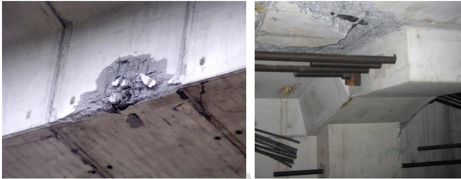
Figure 5-10: Pull out concrete due to abnormal duct placement
