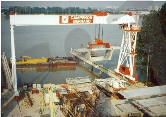
Figure 5-20: Travelling gantry crane
