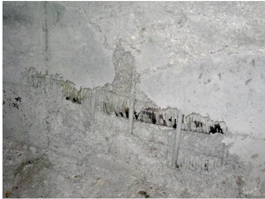
Figure 5-9: Lack of cover of reinforcement
