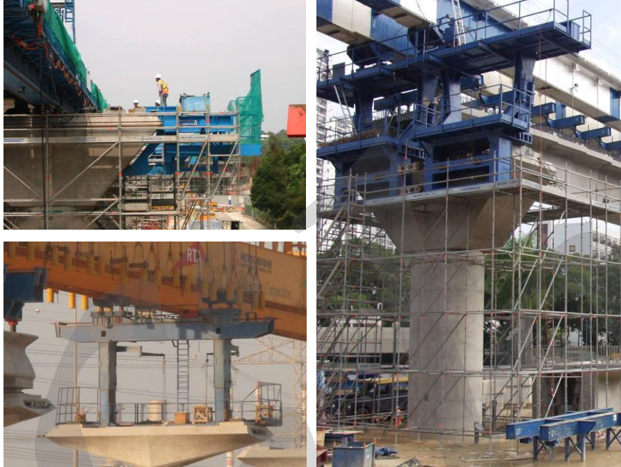
Figure 5-40: Top left: support bracket for underslung girder; bottom left: front support of overhead girder above pier head; right: access and front support for overhead girder
