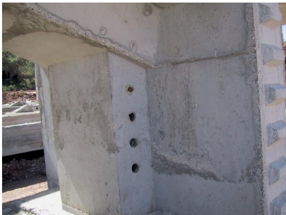
Figure 5-7: Grout leakage due to formwork leakage
