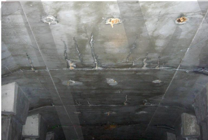
Figure 5-11: Cracking due to local stresses at the segment interface
