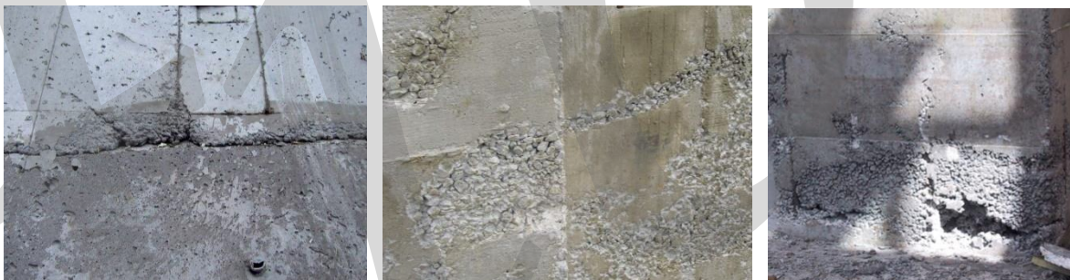
Figure 5-8: (from left to right). Cold joint, honeycomb, and lack of concrete compaction in segments
